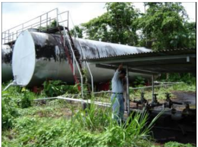
Fuel bunker at Wakay with missing pumps to transfer fuel to fuel tanks of the pumps.
