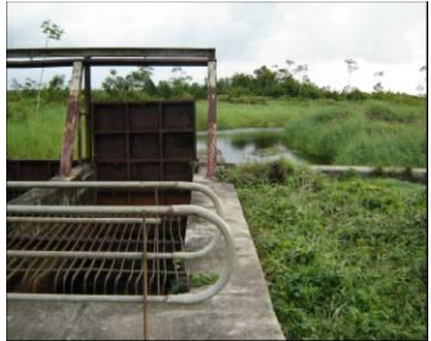
The Inlet sluice at IKUGH. The sluice doors are not functioning properly, however fundament of the construction in good condition.
