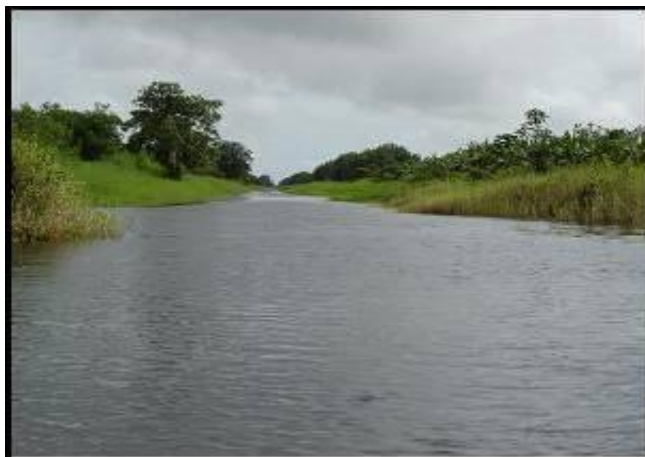
A view at the end of the Corantijkanaal, nearby the Nanni sluice looking relatively good maintained.
