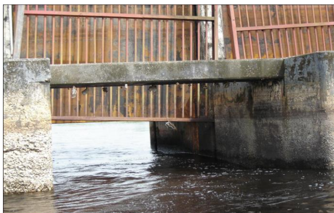
The Nanni sluice of the Nanni inlet. The fundamentals looks good but the trash hark is missing and the doors are not functioning well.
