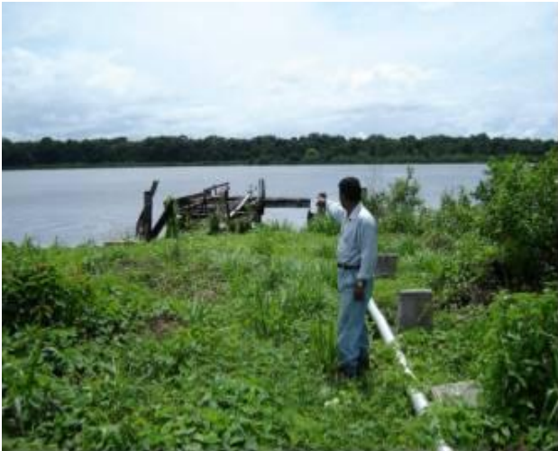
Mr. Padarath, technical assistant at the Wakay puming station, shows the Scaffold, arrear in maintenance. Tankers (fuel boats) can hardly moor here.
