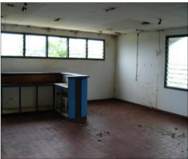
Destroyed office room in the building of the Wakay pumping station.
