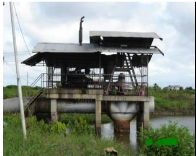
An old pumping installation at the Kaaiman polder (Wageningen) providing irrigation water to the immediate rice fields and in the past also to the "Middenstandspolders" (middleclass farmers).
